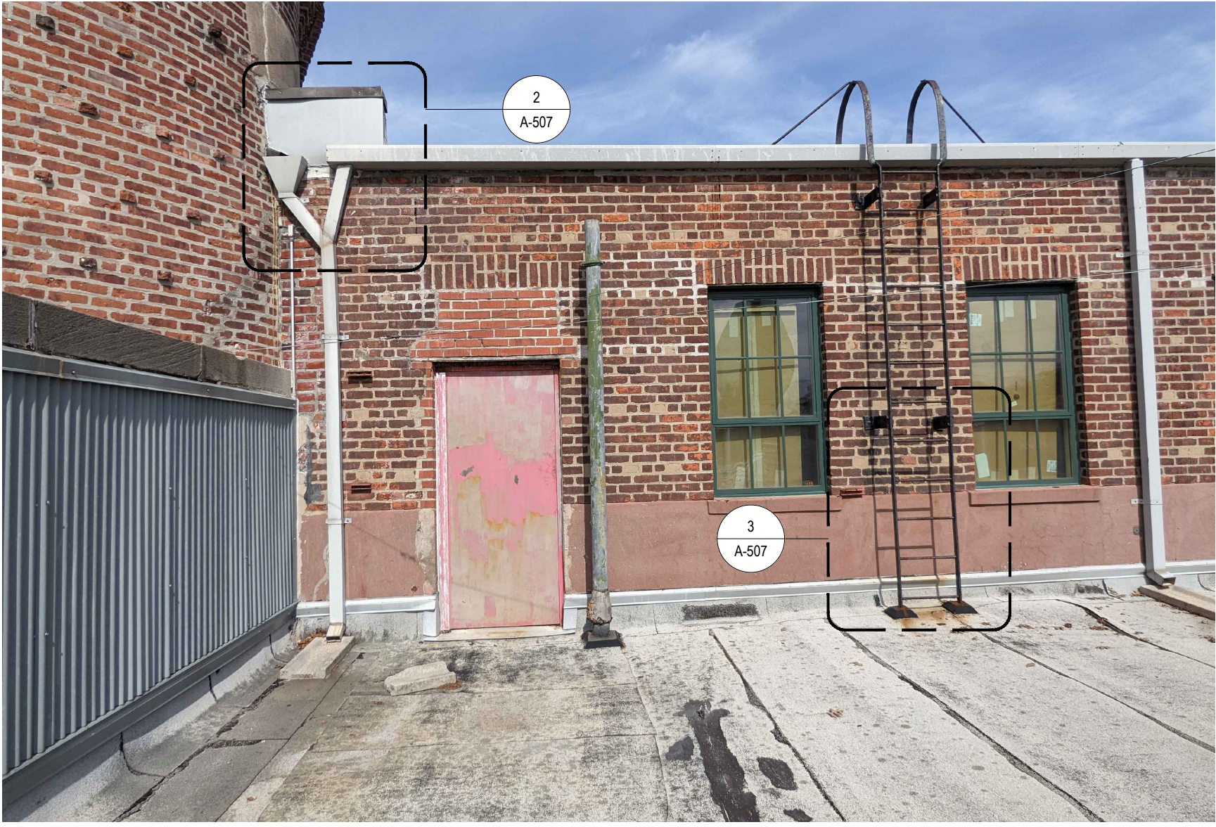
1 ROOF A DRAINAGE & FIXED LADDER FROM ROOFS A TO C REF: 1/A-001 SCALE: NTS
